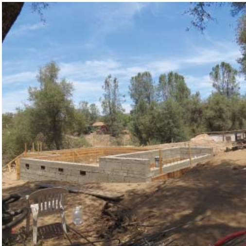
2. The foundation walls are completed. Seen on one wall are four ventilation holes into the crawl space which is where the HVAC system and plumbing pipes will be located.
