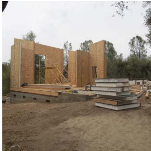
5. The north back wall and north-west corner are up. In the foreground a stack of SIPS panels await placement. Each panel is made of a special foam material sandwiched between two large sheets of plywood. The strength and insulation values are exceptional.
