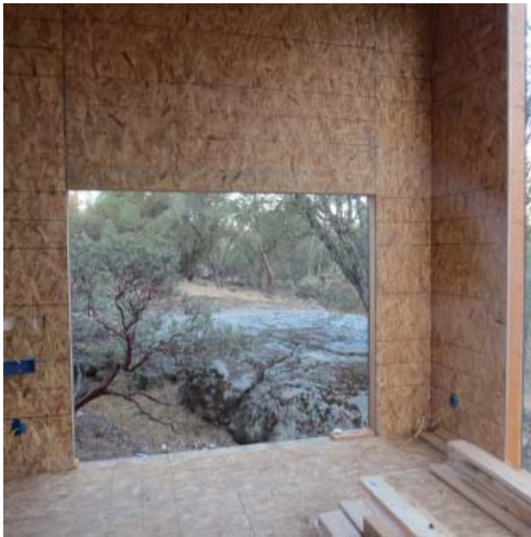
11. Next is a shot of an opening where patio doors will open to a deck that will spill out over a boulder area.
