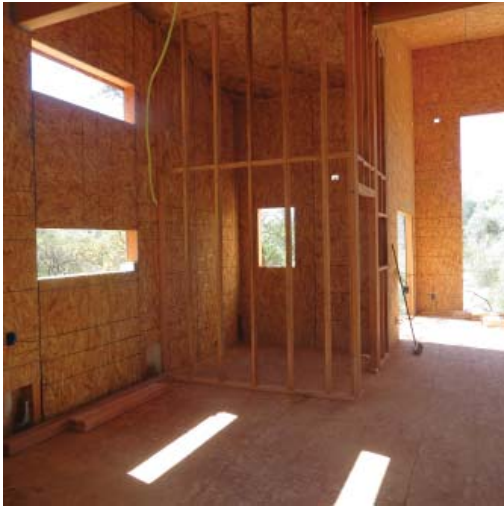
10. Upon entering the building, the inside will be shown, moving in a clockwise direction. The first shot is of the west wall where the kitchen will be located. Adjacent is the wall framing for the bathroom.
