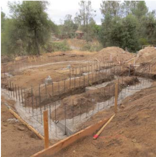
1. The first pouring of the concrete for the supporting walls has been done; re-bar can be seen sticking up, awaiting the second pour.
