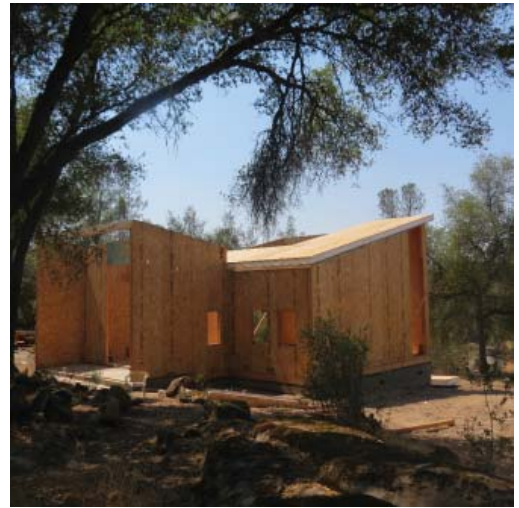
8. This view of the south-east corner shows the front entrance on the left. The main gathering room is on the right, where the highest floor to ceiling distance is about 18 feet.
