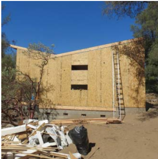
7. Here is the west wall, which will be finished with a natural stone façade. SIPS panels for the roof are in place.
