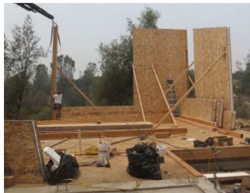
4. The walls of the north-east corner are up. A SIPS (Structural Integrated Panel System) is being used for the floor, walls, and roof. You can see the special crane being used to place the SIPS panels into position.
