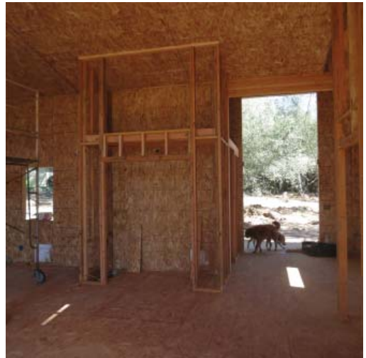
14. In the middle of the south wall, the framing is for a storage closet; the front entrance can be seen on the right
