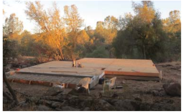
3. The sub-flooring has been laid. The floor-plan footprint is two overlapping squares. The larger square on the right is the main room that will be for gatherings and dining. The smaller square on the left will contain the front entry, kitchen, and bathroom.
