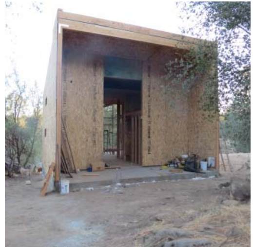
9. This is a straight-on shot of the front entrance. The area outside the front door is a space that will be fronted by 2" x 2" redwood stakes hanging from the roof to the floor.
